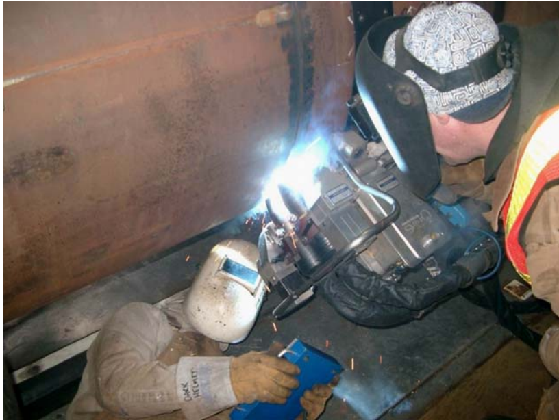
Fig. 8: From four hours per joint to only 20 minutes - these are the sort of welding-time reductions that the TimeTwin Digital system achieves in gas pipeline construction.
