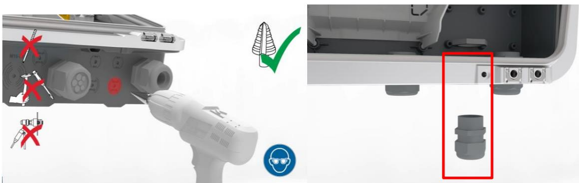
Figure 3: Drilling through the base shell and PG screw fitting inserted at the drilled-through point
