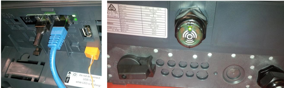
Figure 6. Signal Relay using 12V supply from RJ45 (left) with 12V buzzer mounted to underside of inverter (right)
