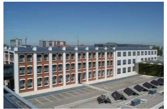
Photovoltaic systems at the Wels site
